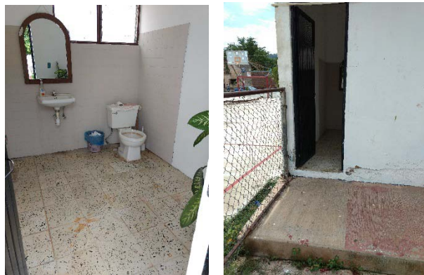
Sanitario – D.I.F. Municipal
